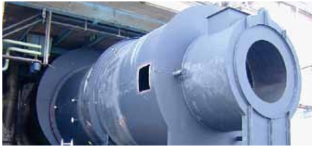
SAACKE hot gas generator during installation
